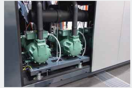
Bearing of HVAC unit with Isotop SD and Isotop FP/K
