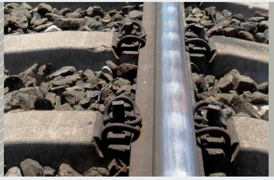
Rail corrugation (long wave)
