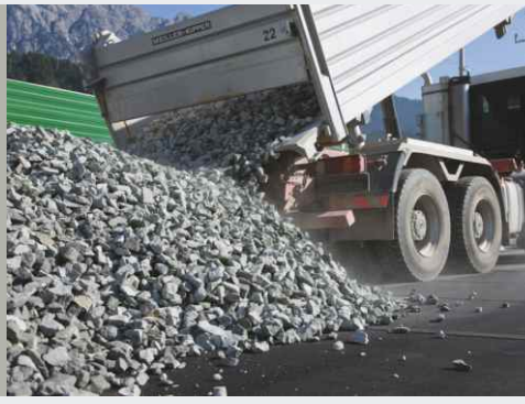
Under ballast mats
