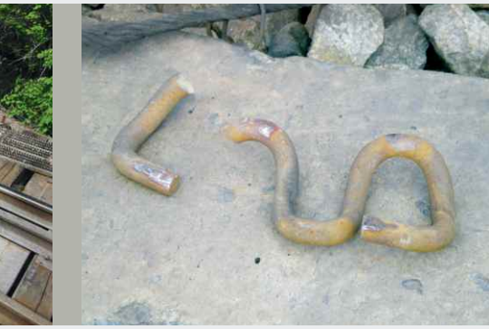
Broken tension clamp
