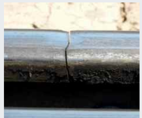
High dynamic forces frequently lead to broken rails.
