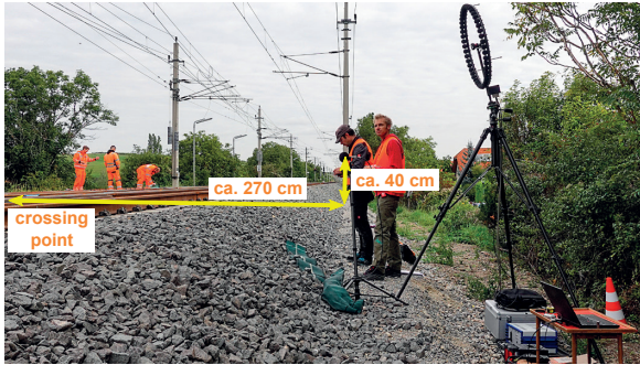
Fig 8. Setting up the measurement equipment to record the noise of passing trains during the field trials at Pfaffstätten.
