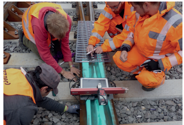
Fig 7. Voestalpine staff checking the turnout crossing geometry at Pfaffstätten prior to the in-track noise measurements being recorded.
