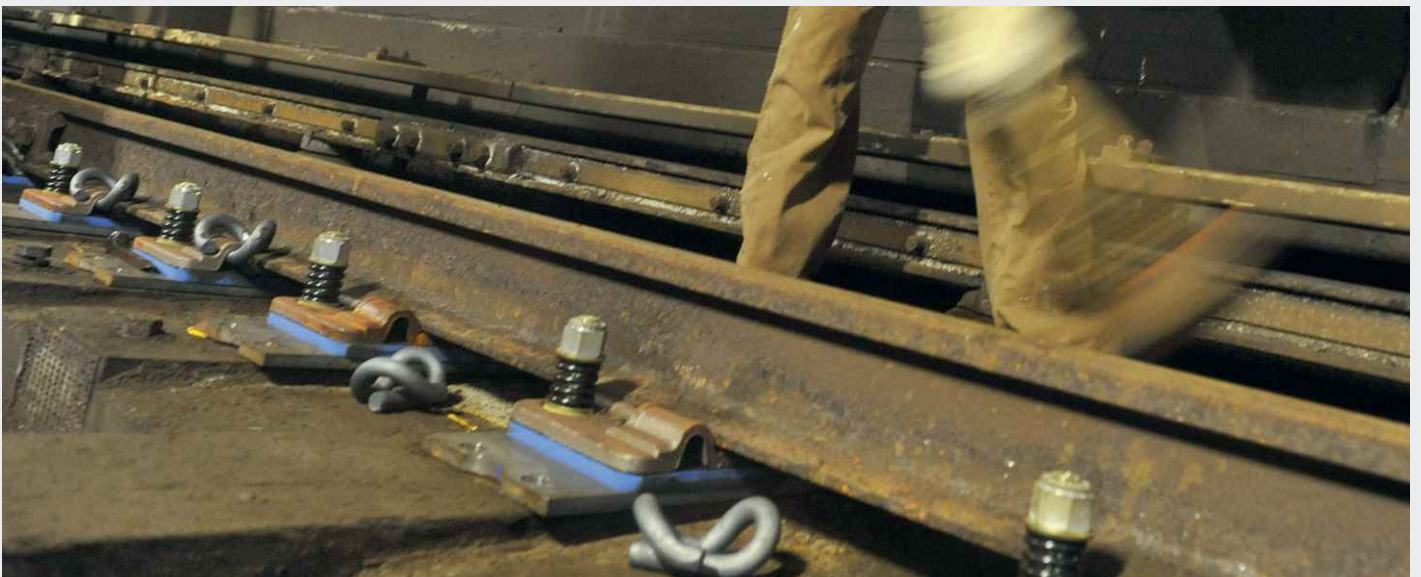
Installation of baseplate pads in the NYC Transit subway system – in use for 20 years
