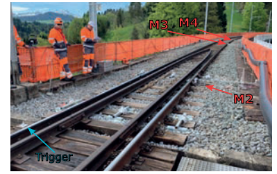
Fig 7. The measuring setup in the field before restoration. Points M2, M3 and M4 are deflection measurements. The role of the trigger is to start the measurement automatically.
