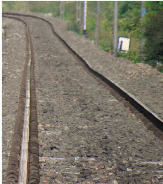
FIG. 15: The differing quality of comparable sections of track is obvious, with under-sleeper pads (left) and without them (right)
