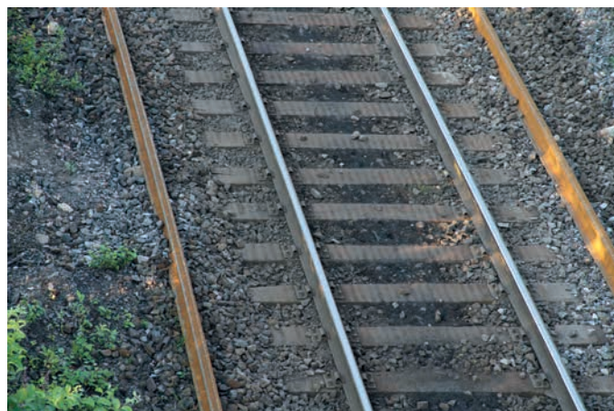
FIG. 5: The line between Gällivare and Koskullskulle equipped with wooden sleepers before renewal
