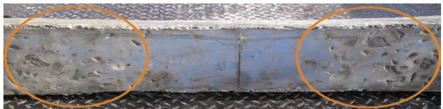
Figure 2: Padded sleeper after 190 million load tonnes with indentations in the Sylomer® material
