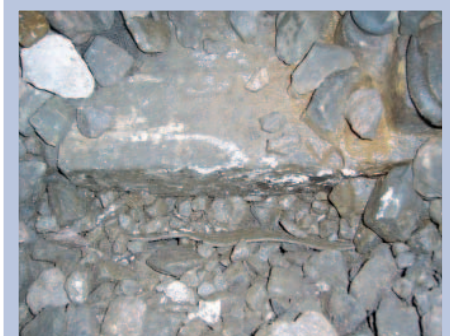
Fig. 2: Removed wooden sleeper with damaged mounts
