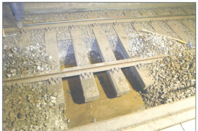
Fig. 1: Two pictures showing exposed under-ballast mats – on the surface, the presence of water is clearly visible
