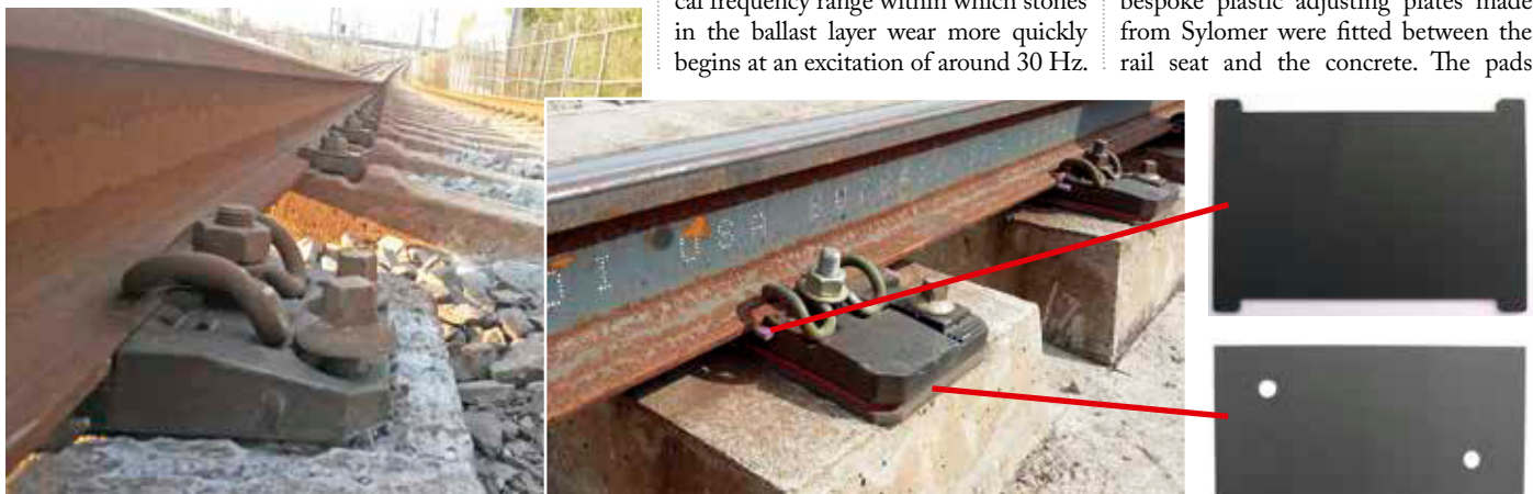
Fig 6. Damage to slab track with loosened fastening bolts (below) can be resolved by installation of plastic compensating plates and elastic rail pads (centre, right).
