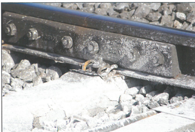
Fig. 5: Formation of white spots at an insulated rail joint
